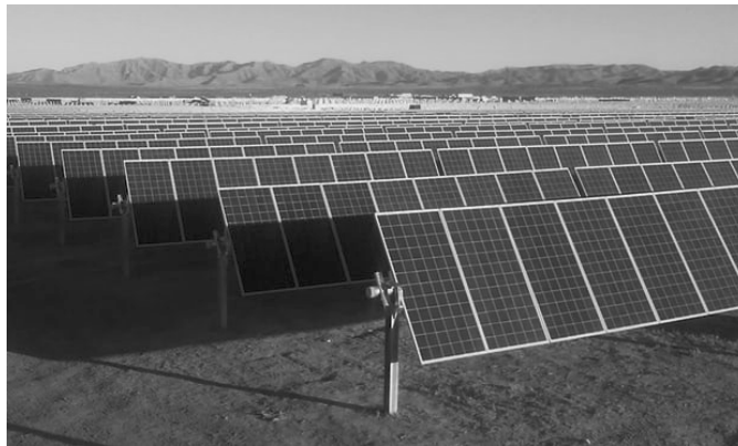
Fig. 3. A solar energy plant in Oklahoma
